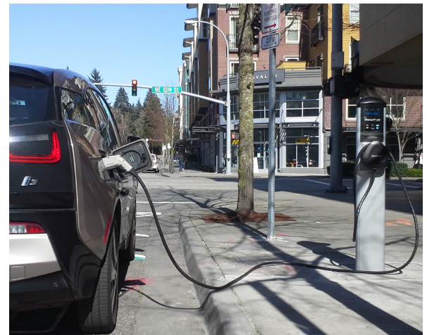
Electric vehicle charging station
